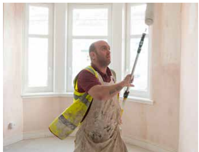
Work progressed in refurbishing private acquisition flats for social renting and mid market rent.
