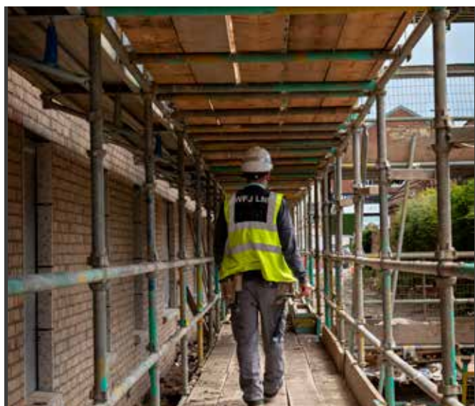
On site in Admiral Street with CCG Ltd building 35 new affordable homes.
